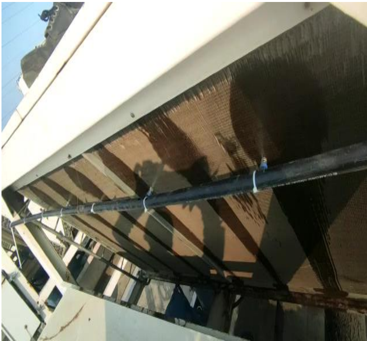
Misting / Precooling will improve chiller efficiency
